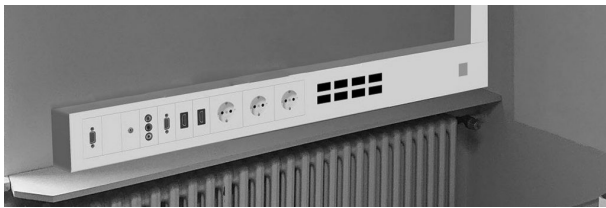
Figure 6: Photomontage of how the integrated control unit should look like. Video connections, sockets, the control unit and a main switch are integrated directly into the 50 mm device installation channel.
