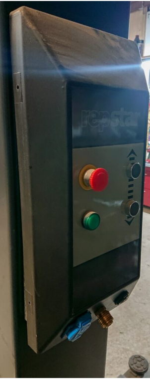
Lift control unit (with 230 VAC and 12 VDC supply)
